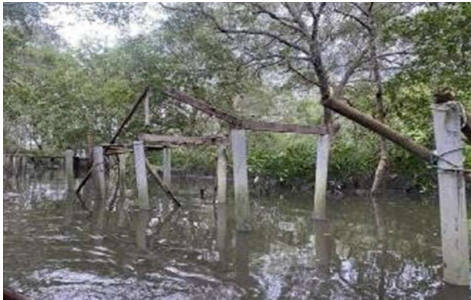
Figure 2 Damaged Ecotourism Facilities (bridge)
